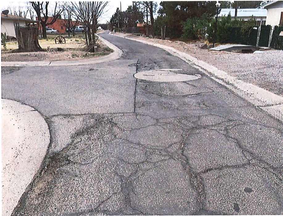
Photo 3. Calle de Colon – Current Road Condition – West view at Calle Cuarta intersection
