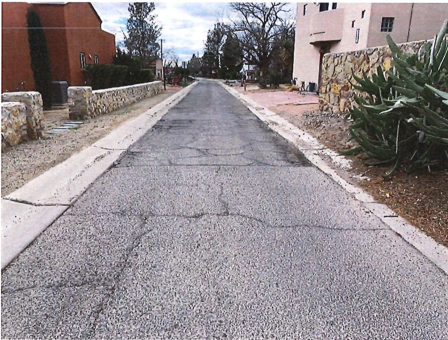
Photo 6. Calle de Colon – Current Road Condition – West view near Calle Tercera
