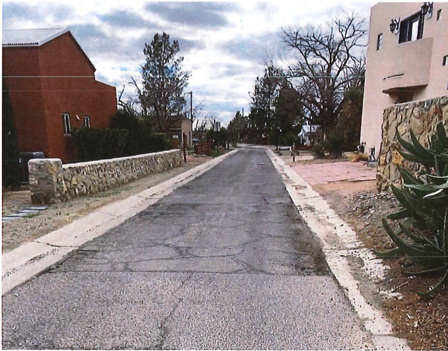
Photo 5. Calle de Colon – Current Road Condition – West view near Calle Tercera
