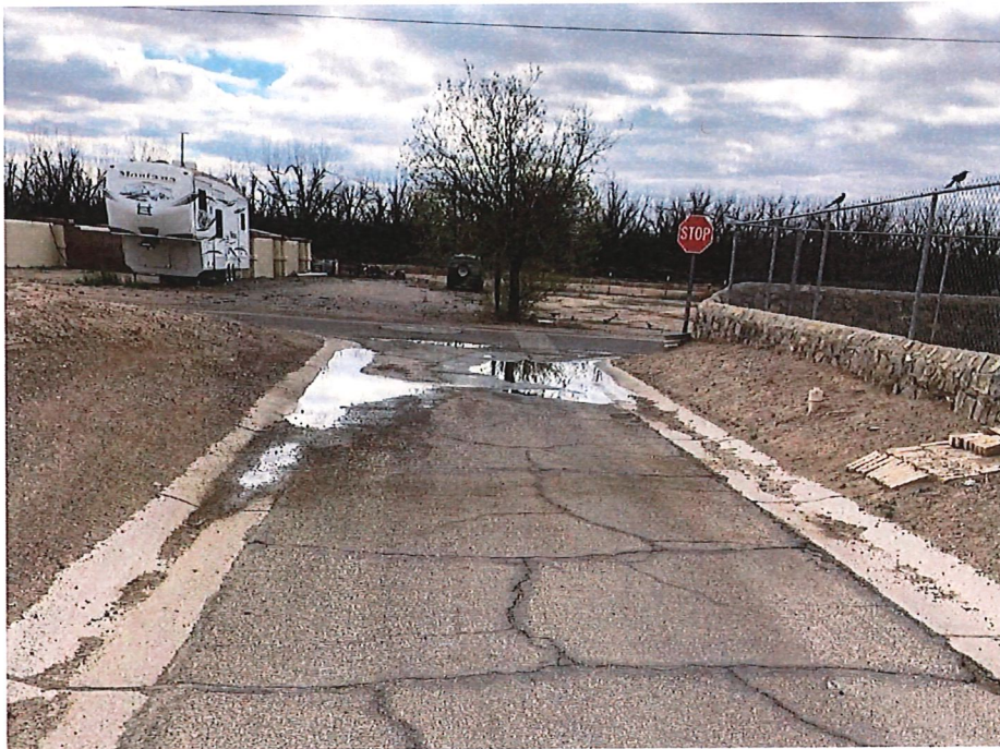
Photo 8. Calle de Colon – Current Road Condition – West view near Calle de Oeste
