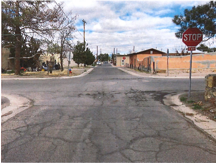
Photo 9. Calle de Colon – Current Road Condition – East view near Calle Principal
