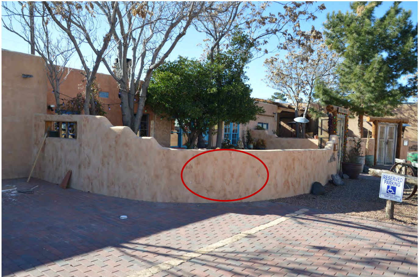
PHOTO OF THE SUBJECT WALL FROM CALLE DE SAN ALBINO
