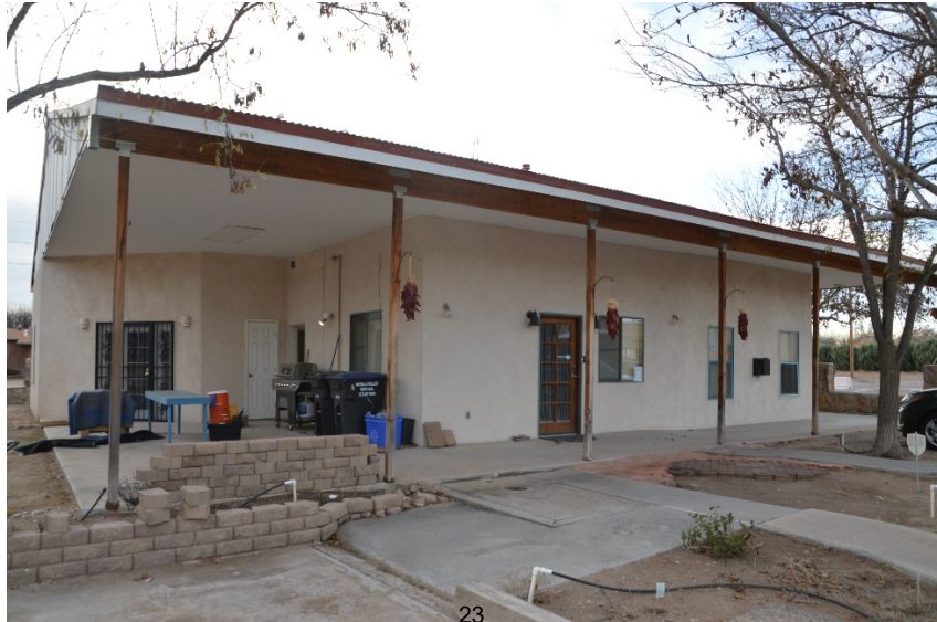
PHOTO OF PORCH SHOWING POSTS TO BE REPLACED
