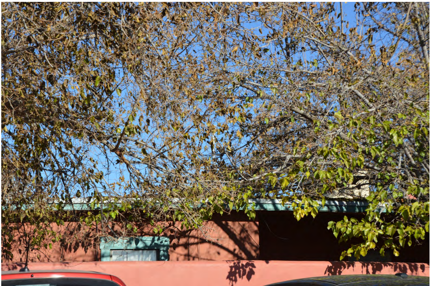
PHOTO OF PROPERTY FROM ANDELE'S DOGHOUSE SHOWING FACIA BOARDS
